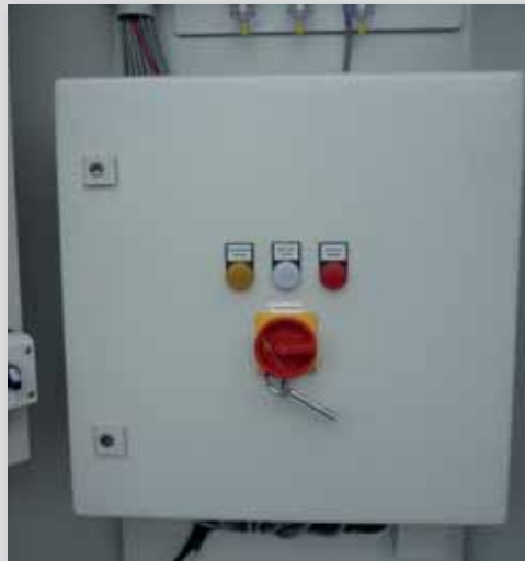
Central control unit
