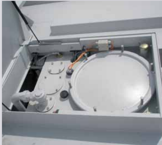
Hood with equipment
