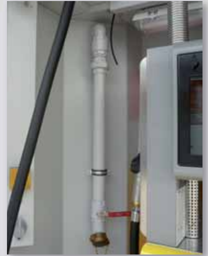
Tank vehicle filling connection
